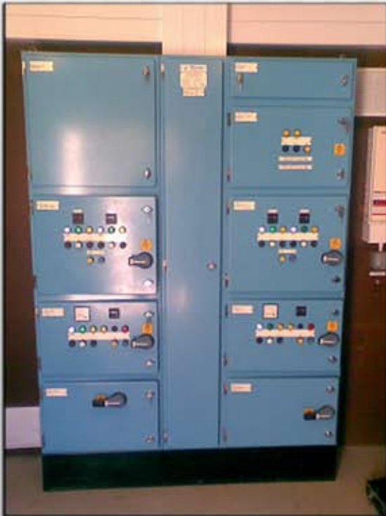
Motor Control Centre
