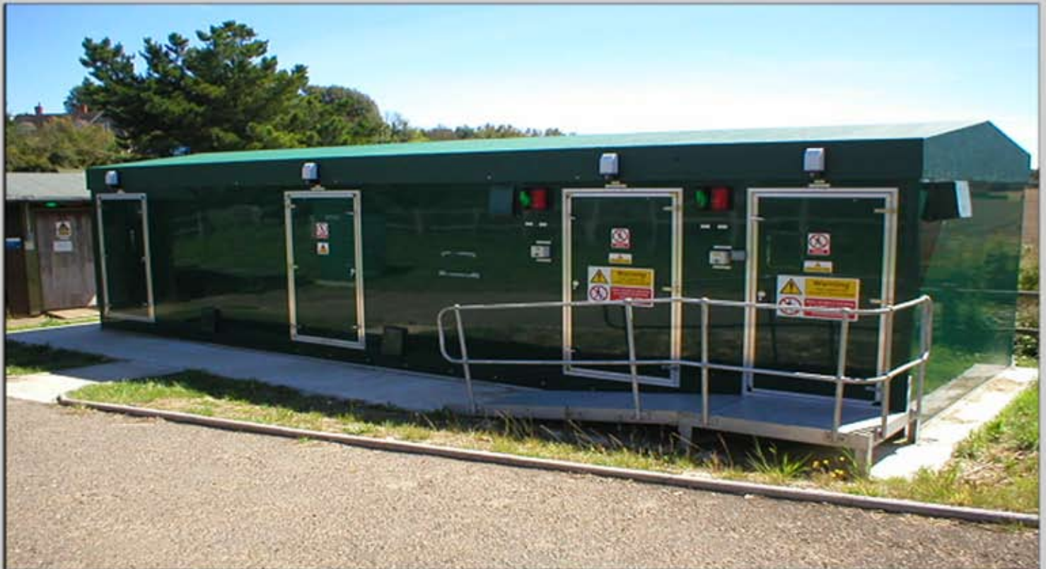
Site: Clapham Disinfection Kiosk - Internal View
