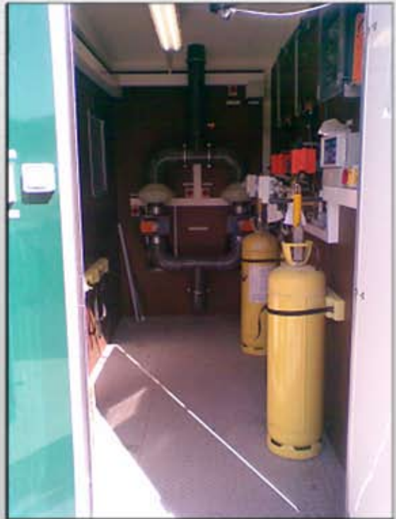
Secondary Disinfection Gas System
